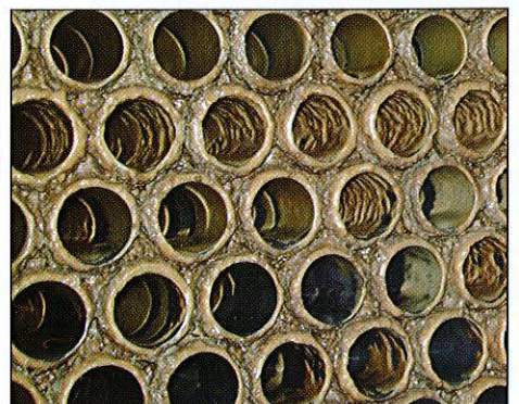
Scale Build-up on Tubes
