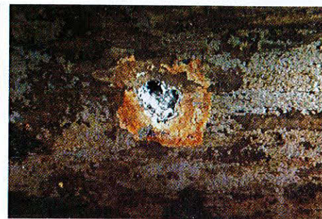
Under Deposit Corrosion - Pitting Due to Manganese Deposit
