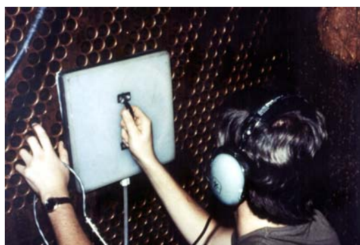
Figure 14 Technician with Plenum
