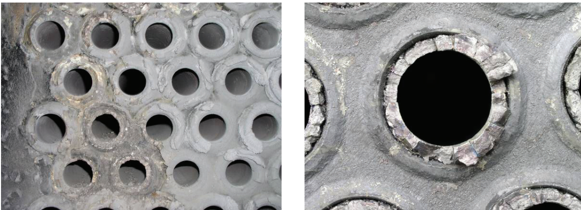
Figure 7. Tubesheet and tube internal with 0.32" iron pyrite deposit before LN2 cleaning
