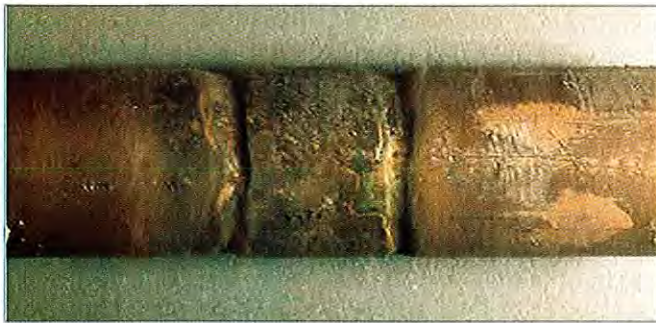
Figure 7: Ammonia condensate grooving in admiralty brass tube. Grooves formed on each side of tube support plate.
