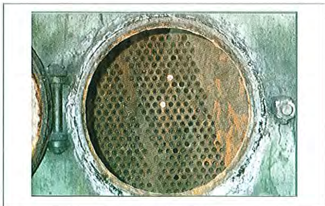
Figure 4: View of inlet-end tubesheet through manway; tubes are filled with microbiological slime that is dried and flaky.
