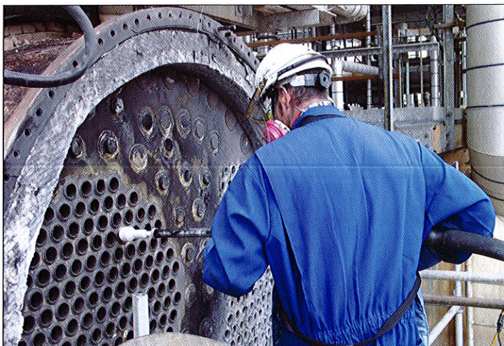
NitroLance Cleaning Tube Sheet
